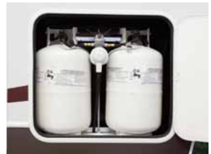
■ Easily accessible 30 lb. propane gas cylinders with auto changeover, and at the right height. No bending over!
