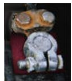
Clean, Maintained Battery Cable Terminal
