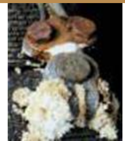
Corroded Battery Cable Terminal
