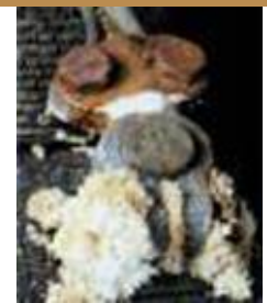
Corroded Battery Cable Terminal
