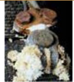
Corroded Battery Cable Terminal
