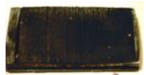
Extremely Dirty/Restricted Air Filter
