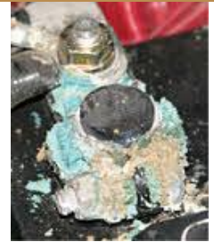
Corroded battery terminals
