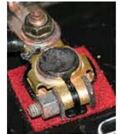
Battery terminals after service
