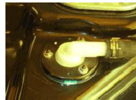
A dye test can determine the exact point of the leak
