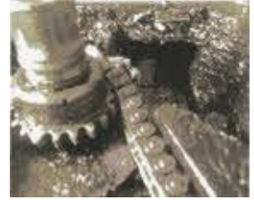
Sludge from lack of oil changes
