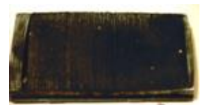
Extremely Dirty/Restricted Air Filter
