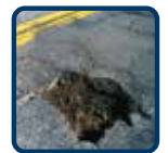
POTHOLES/ DAMAGED PAVEMENT
