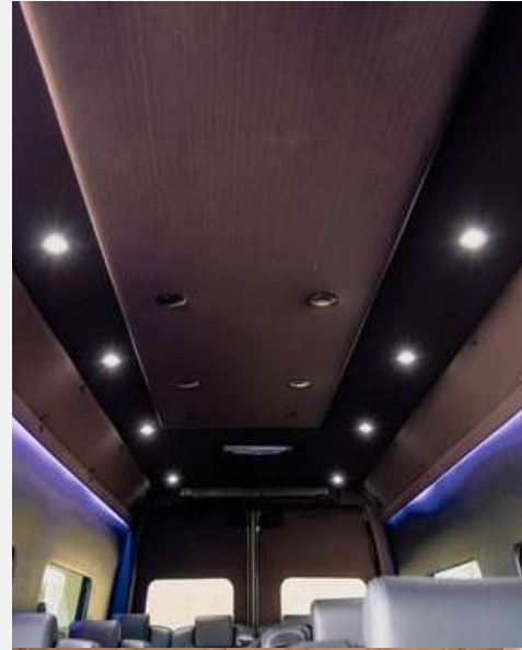
Recessed Lighting Fixtures
